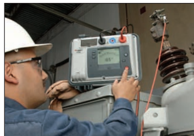
Circuit breaker being tested with the S1-552/2
